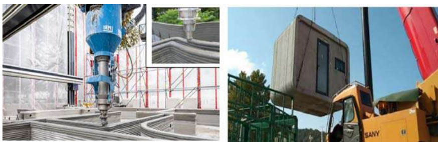
Fig. 1 (a) Concrete 3D Printing Nozzle (b) 3D printed isolation wards for COVID-19 using concrete [Courtesy: Winsun 3D Printing].
